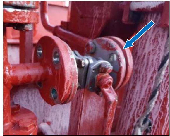
Figure 5: Right flange: location where sulphuric acid allegedly sprayed out from (blue arrow)
